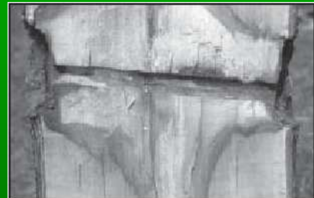
Figure 2. Some years after installation of a crown anchor: The bolt with a diameter of 18 mm (0.7 in.) led to discoloration and white rot above and below the drill hole.
